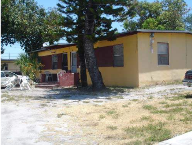
Figure 27: Lack of property maintenance
