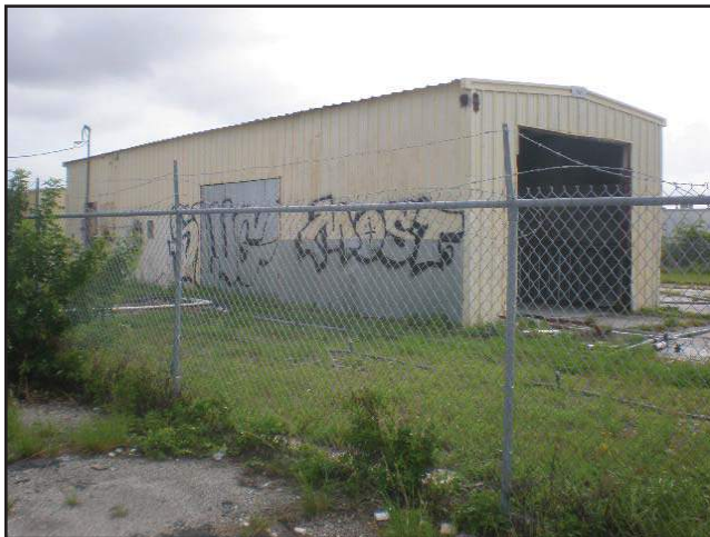
Abandoned structure, vandalized
