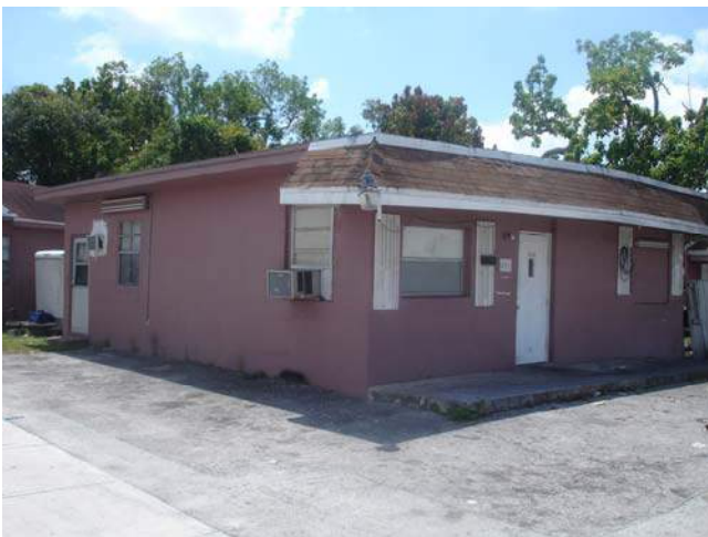
Figure 16: Deteriorating multi-family structure with inadequate parking and landscaping
