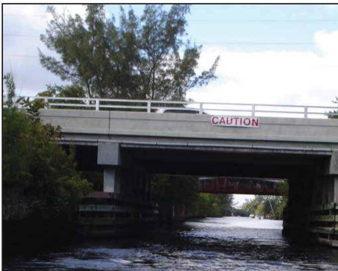
Low bridge height at Cut-off canal
