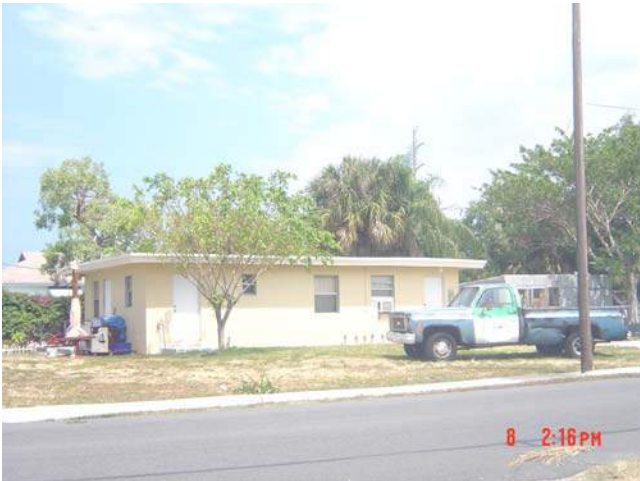
Figure 25: Inadequate off-street parking, deferred maintenance
