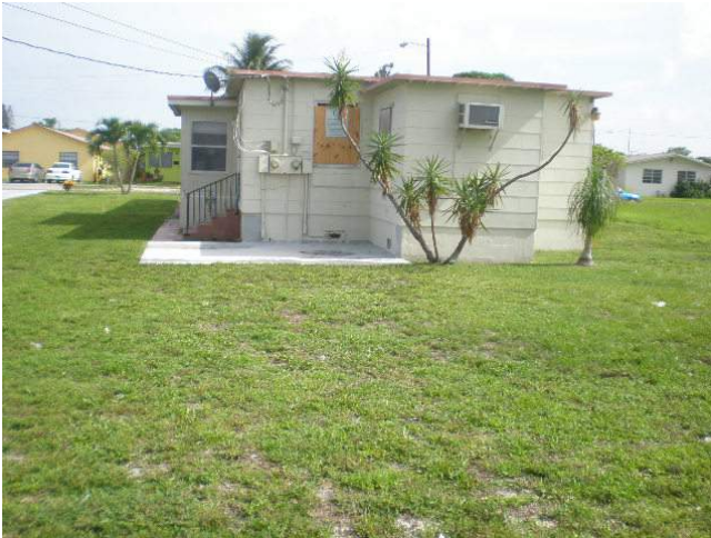
Figure 21: Boarded up windows
