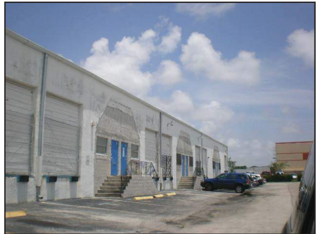
Deteriorated commercial and industrial buildings
