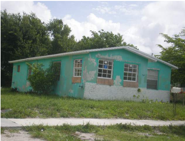
Figure 9: Deteriorating structure, lack of maintenance
