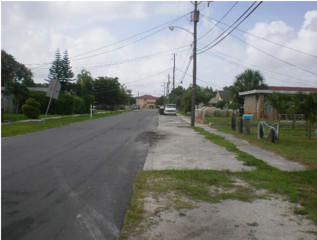
Figure 3: Unfinished infrastructure lacking swale and sidewalk maintenance
