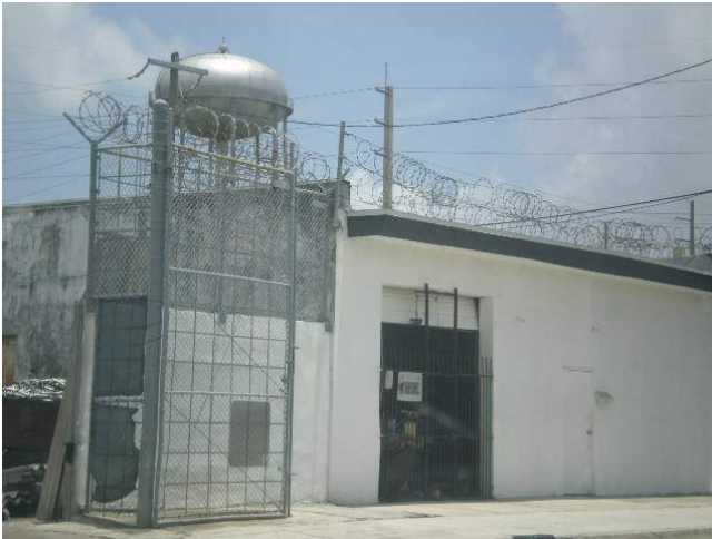
Figure 32: Deteriorating industrial property
