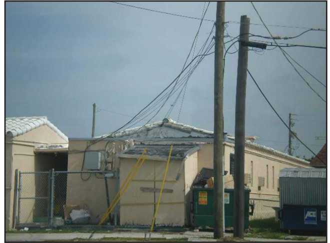
Unsafe structural and infrastructure conditions – obstructions in walkway
