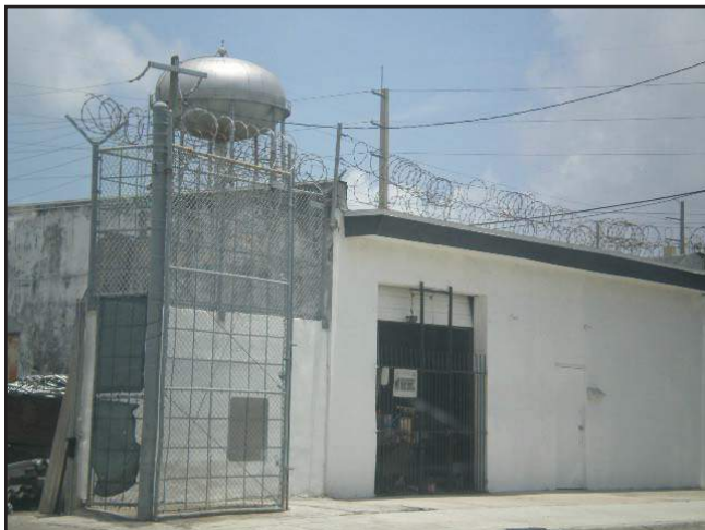
Deteriorating industrial property
