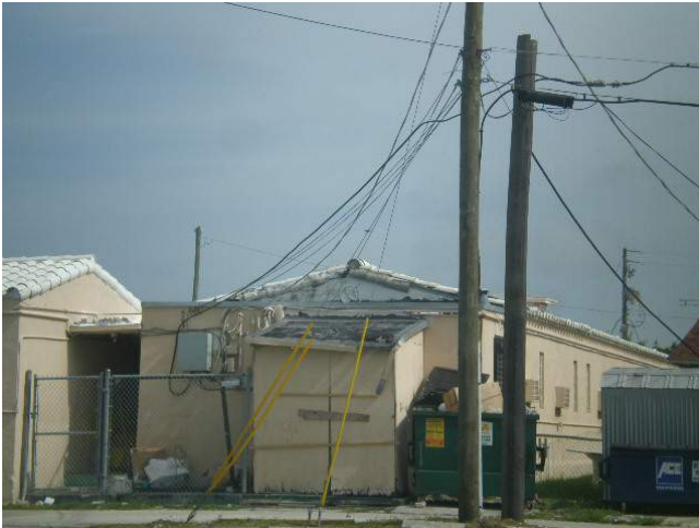
Figure 6: Unsafe structural and infrastructure conditions – obstructions in walkway
