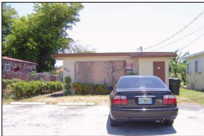
Lack of maintenance; need safer structures
