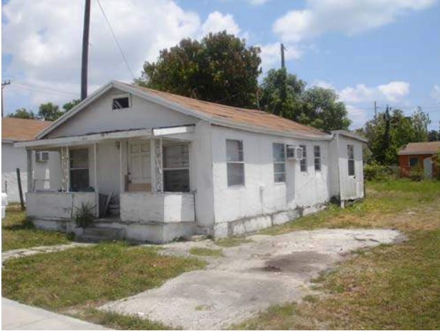
Figure 17: Aging, dilapidated structure, unsafe site conditions
