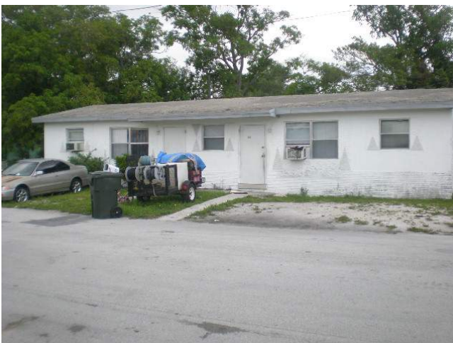
Figure 4: Deteriorating structure and site conditions – inadequate parking
